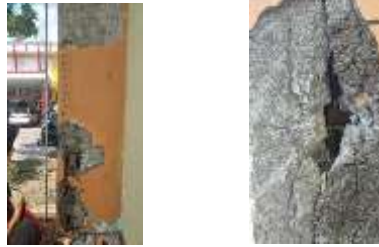
Fig. 1 Condition of the 1st-floor column of the Rectorate Building Muhammadiyah University of Sumatera Barat (Private documentation, 2024).
